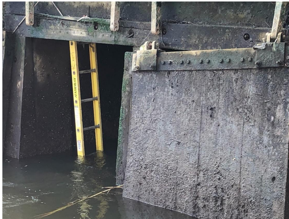
Exhibit A: Late September, 2021. Photos showing the status of Town Line Brook tide gates prior to emergency repair completed by the City of Revere. Click here for video of leaking tide gates at Town Line Brook tide gates.
