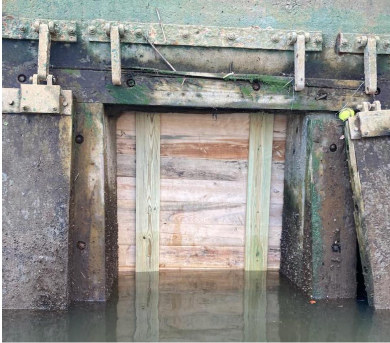
Exhibit B: Late October, 2021. Town Line Brook tide gates after emergency repair completed by the City of Revere.
